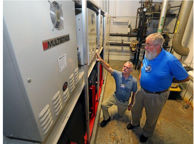
Tim Morris, Assistant Director for Facilities Management (left), points out operating features of the Multistack Heat Recovery Chiller unit at the USA Medical Center to Lawrence Gardner, Director for Facilities Management.
